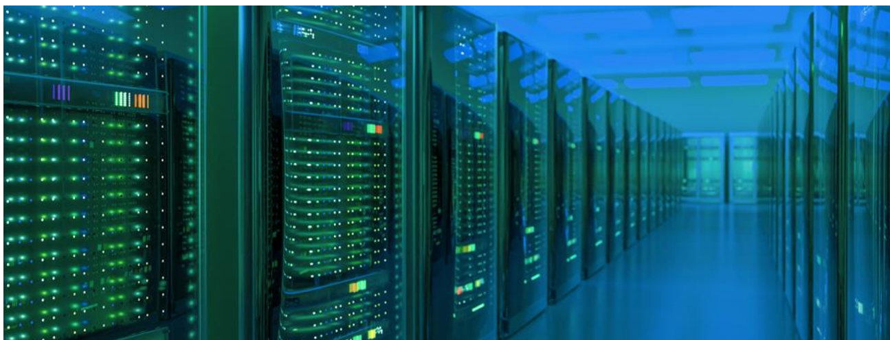
E-house modules for generator sets.
