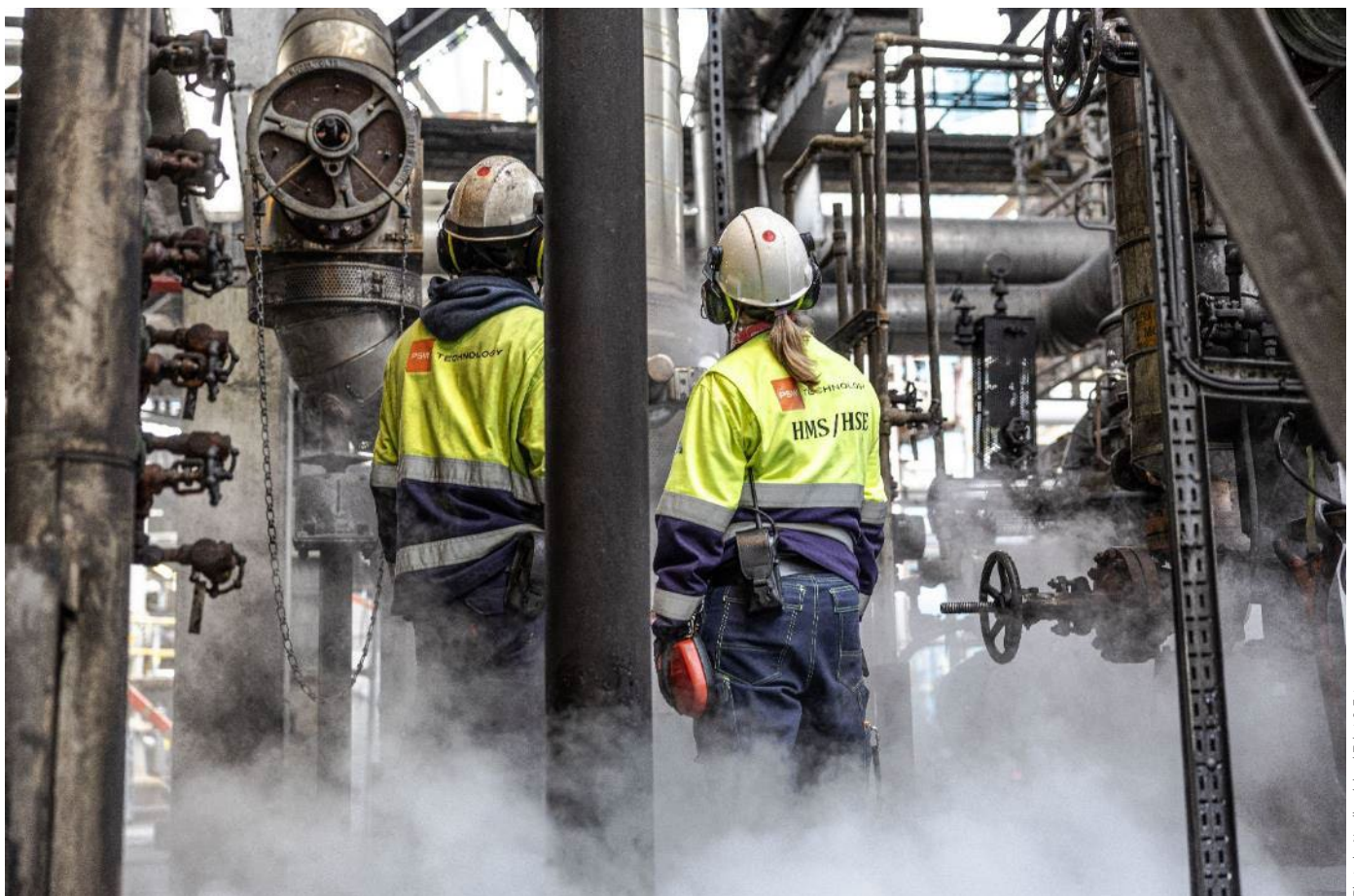
Scana companies deliver a wide range of products and services to the Mongstad Refinery.
