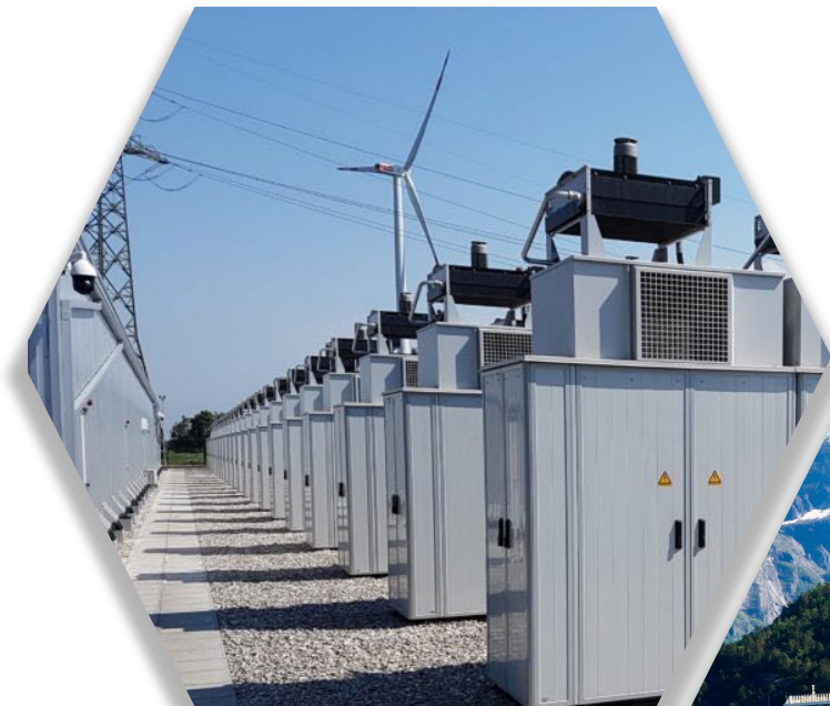
ENERGY STORAGE SOLUTIONS
